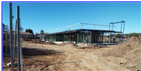
LEARNING CURVE: Construction is well advanced on the new MET Armidale Campus school in Maude St
